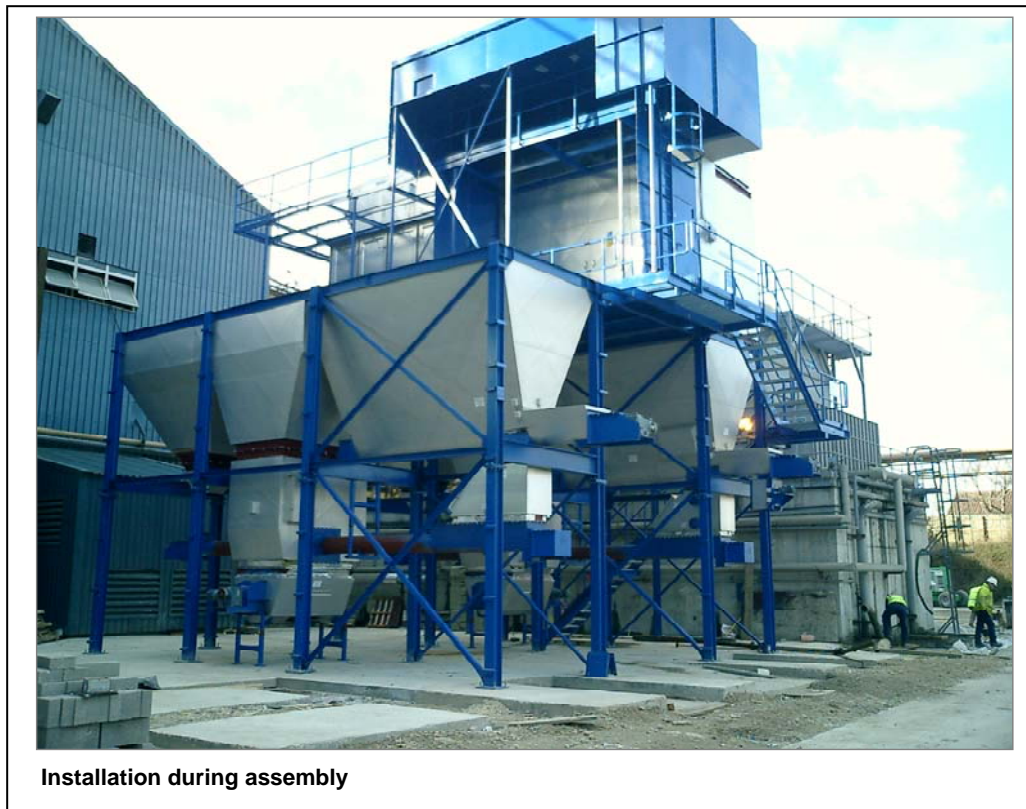
Pic 13: Application example Fabric filter downstream trunk for container glass
