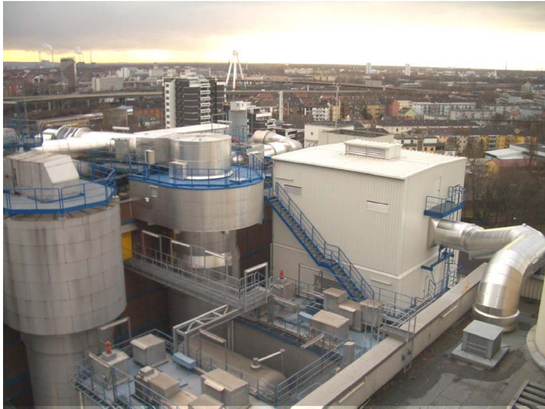
Illustration 2: MHKW Ludwigshafen crude gas cleaning line 2 Spray absorber head and filter / reactor building
